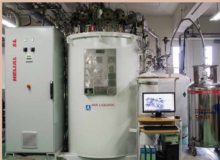
Fig. 1: Helium liquefier in CL
